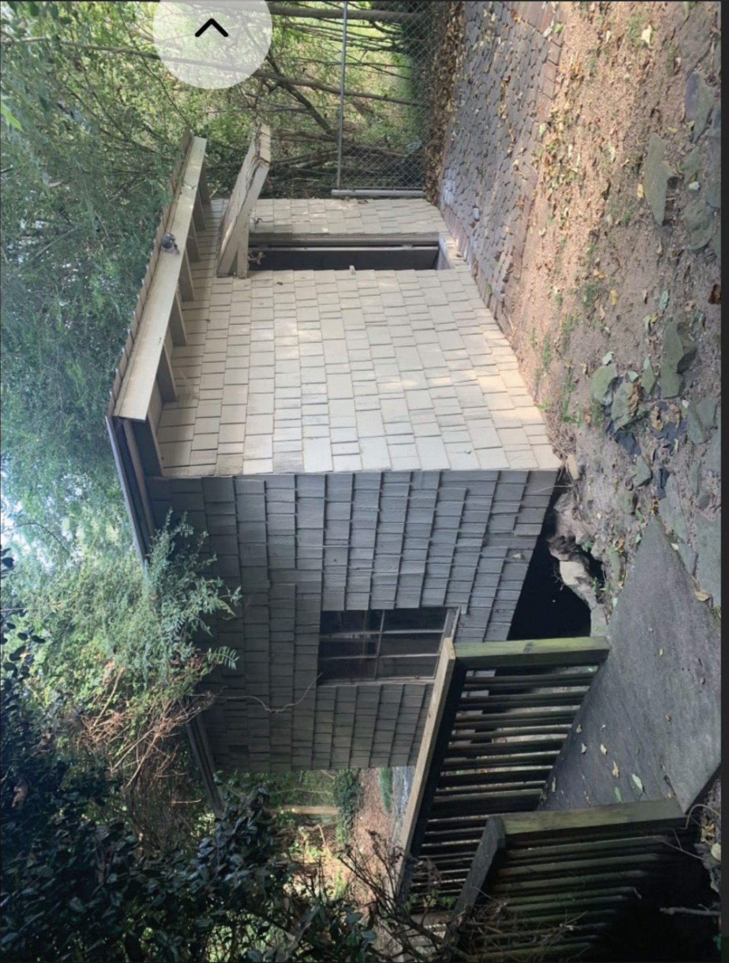
moisture damage, wood decay, fungal growth, broken
